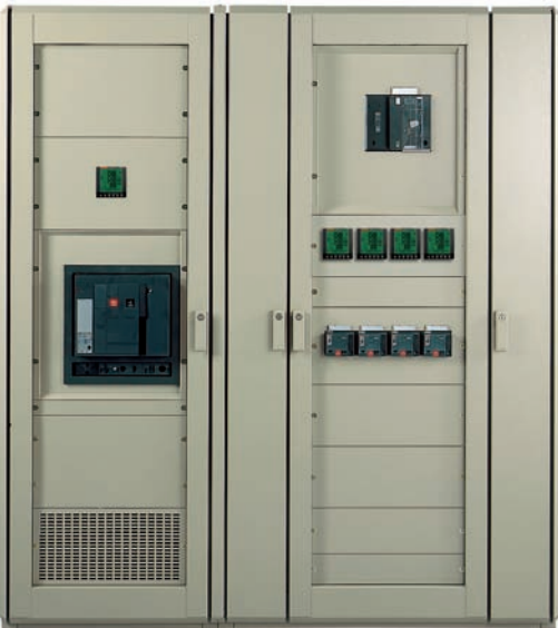
Main LV switchboard.
